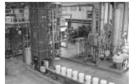
Medical waste moving down the conveyor to be processed by the PAT facility
